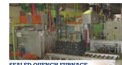
SEALED QUENCH FURNACE
